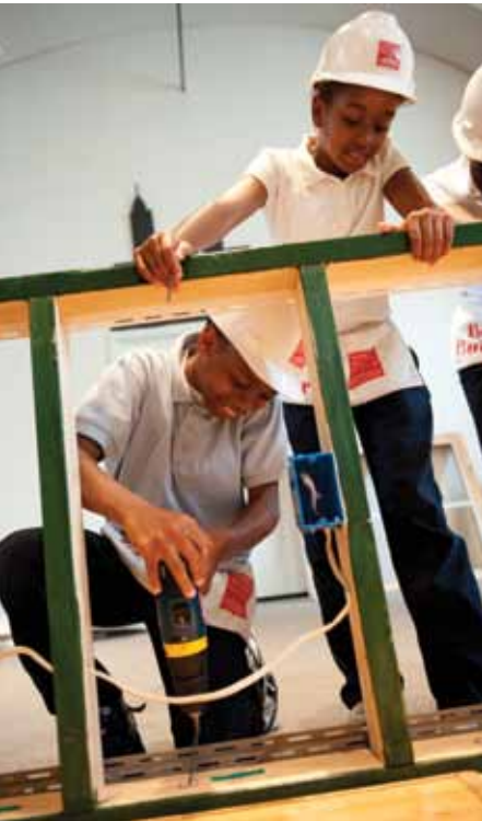
Students join a work crew, become carpenters, and use power screwdrivers as they assemble an 8' x 11' house during the Be a Green Builder school program. Photo by Kevin Allen
